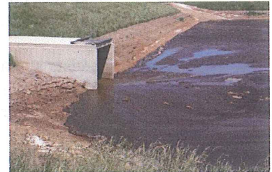
Non-enclosed manure storage should be assessed to determine employee exposure to safety and health hazards.
