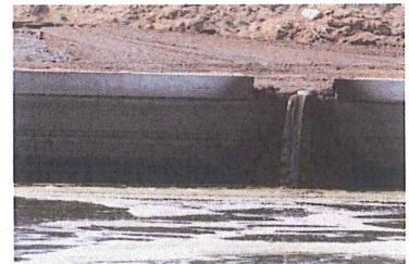
One potential hazard is someone falling into the storage and being engulfed in the manure slurry.
