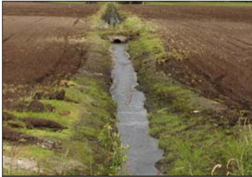
The lack of a vegetated filter strip along this field ditch presents risks of water quality degradation due to erosion and bacterial contamination. The ditch also requires more maintenance at a higher financial cost over time.
